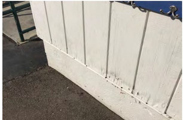
#10 TEXTURED PLYWOOD SIDING WATER DAMAGE
