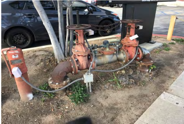
#55 6" FIRE BACKFLOW PREVENTER
