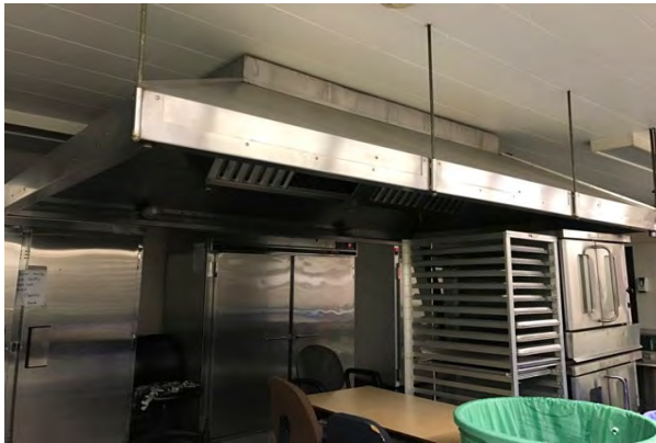
#63 COMMERCIAL KITCHEN EXHAUST HOOD
