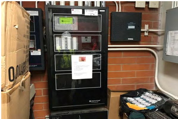
#59 FIRE ALARM CONTROL PANEL
