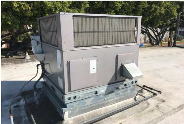
#53 HEAT PUMP (RTU)
