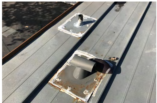
#24 PORTABLE 12 DAMAGED FLASHING SEAL
