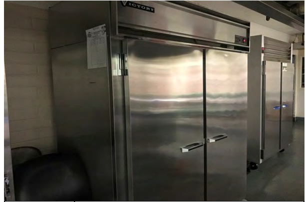
#62 COMMERCIAL KITCHEN 2-DOOR REFRIGERATORS
