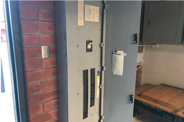
#56 400 AMP DISTRIBUTION PANEL
