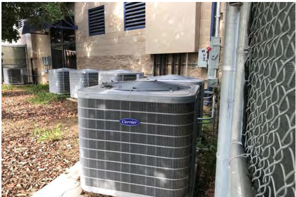
#48 DUCTLESS SPLIT SYSTEM CONDENSER UNITS
