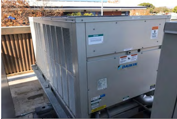
#49 20 TON CONDENSING UNIT
