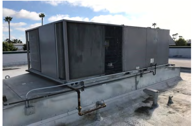
#54 PACKAGED UNIT (RTU)
