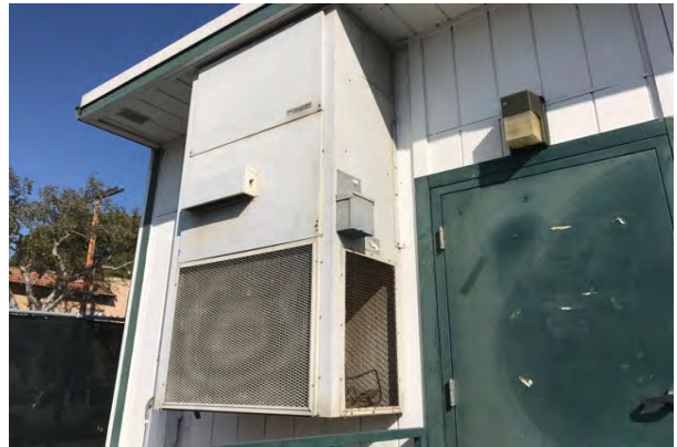
#52 3.5 TON HEAT PUMP
